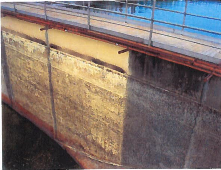
Overview of Warren Environmental S-301-14 material.
