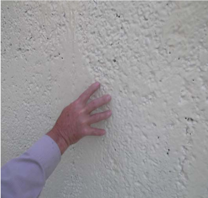
Figure#1: Example of Bug Holes Not Filled with Coating.
